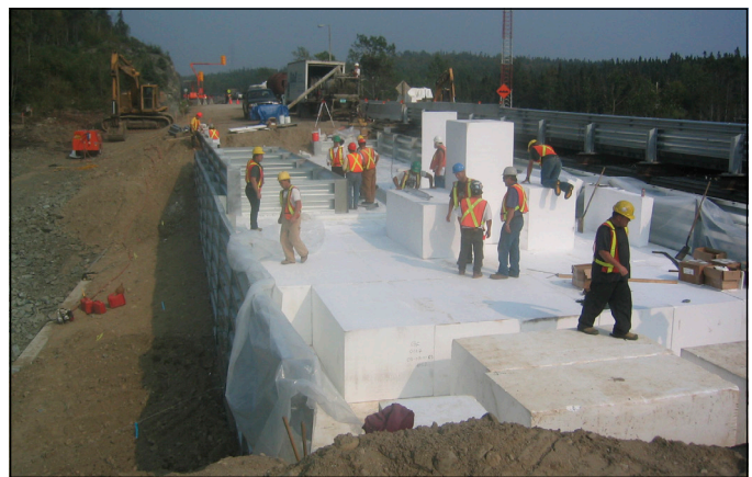
Figure 13—Expanded polystyrene geofoam embankment fill along I-15, Salt Lake City, Utah. Geofoam Research Center, Syracuse University.
