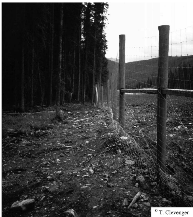
Figure 3. Image of a ungulate-exclusion fence under construction along Phase IIIA. Note the chain link apron attached to the bottom of the page wire. Eventually the bottom 1 m of the apron will be buried.
