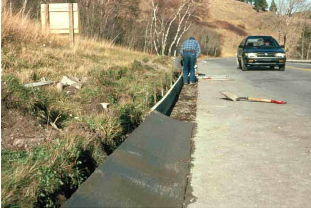
Figure 59. Photo. Construction of amphibian ramp to replace curb and allow cross-road movement of long-toed salamanders (Credit: Parks Canada).
