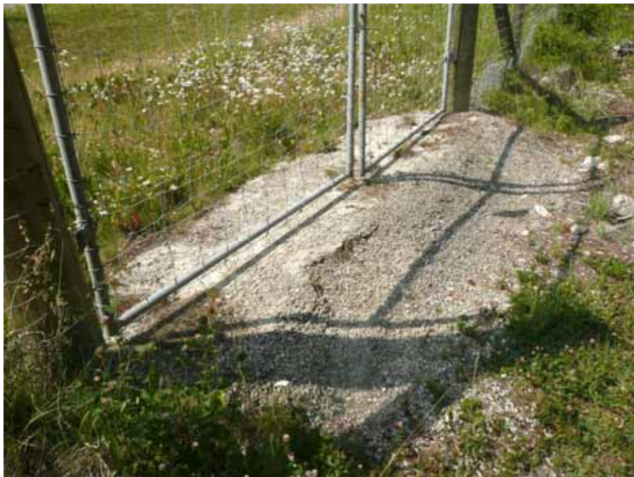
Figure 66. Photo. Concrete base of swing gate to prevent animal digging under wildlife fence (Credit: Tony Clevenger).
