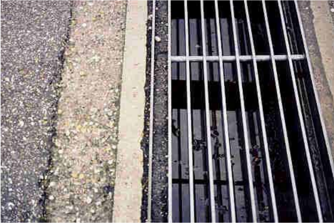
Figure 57. Photo. Grated slots on amphibian tunnels allows light and conservers ambient temperatures and humidity (Credit: Anonymous).
